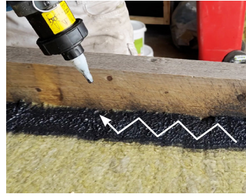
Spray layer 2 in a zig-zag pattern. Spray very close to the edge (but not up the edge)
