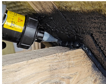
In caulking mode, place a bead around the collar beam/rafter shoe. Make sure there is enough sealant for the vapor barrier to be pressed into it.
