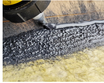
Using caulking mode, run a bead along the edge. Make sure there is enough sealant for the vapor barrier to be pressed into it.
