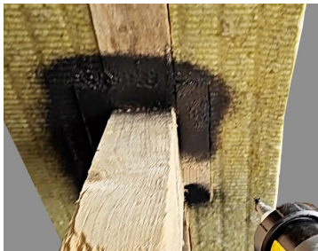
Spray a 10 cm wide strip at least 1.3 mm thick around the collar beam/rafter shoe with the nozzle about 20-25 cm from the surface.
